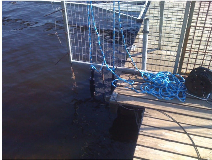
Figure 31 Installation of the probes in Tuppurala
